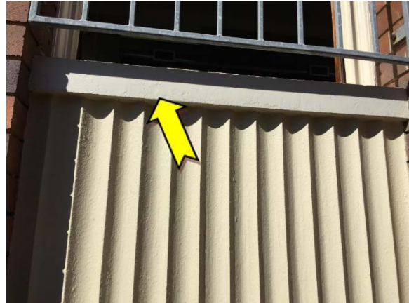
Photo 8. Exterior, throughout, window frames – suspected lead-containing cream upper paint system.
