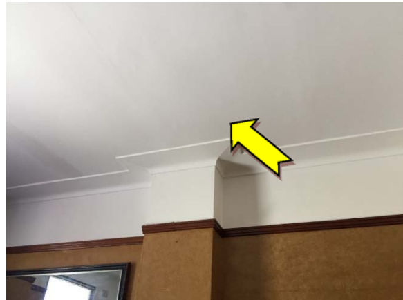
Photo 10. Interior, throughout, ceilings– suspected lead-containing white upper paint system.
