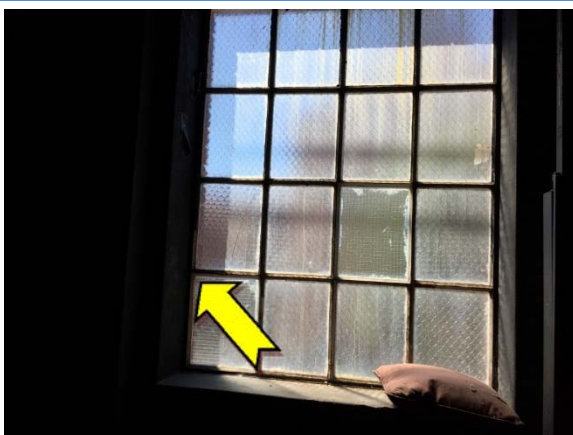
Photo 5. Interior ground level, main hall stage, window frames – non asbestos-containing window caulking.
