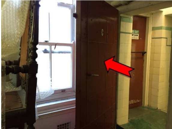
Photo 1. Interior, basement level, fireproof storage room, door core – suspected friable asbestos-containing fire door core.
