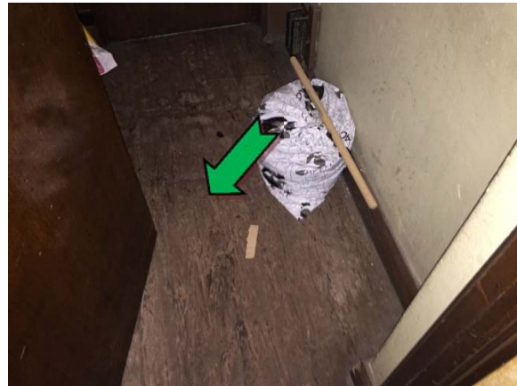
Photo 4. Interior, ground level, store room adjacent amenities room, brown floor covering – non asbestos-containing vinyl floor tiles.
