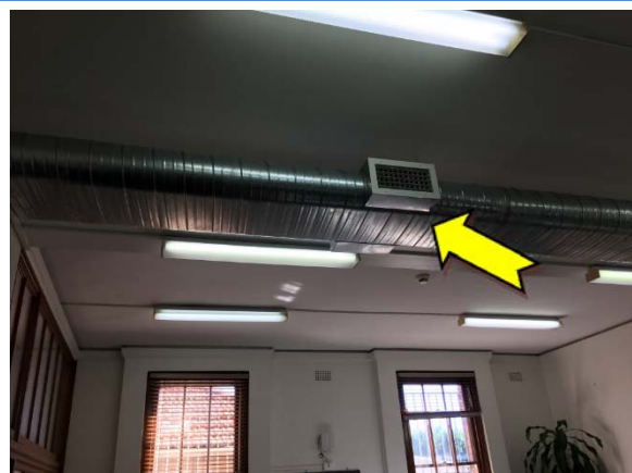
Photo 6. Interior, ground level, throughout, ductwork – suspected SMF internal insulation.
